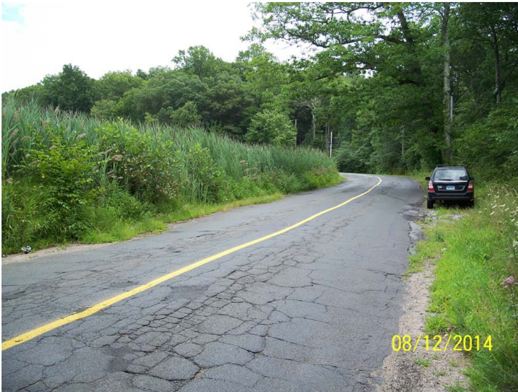
Photo 21k – The emergency overflow area along Hidden Lake Road, approximately 1,200 feet east of the main dam embankment, showing a heavy vegetative growth between the edge of the road and the pond, which edge is approximately 10 feet to the left of the dense growth of phragmites.
