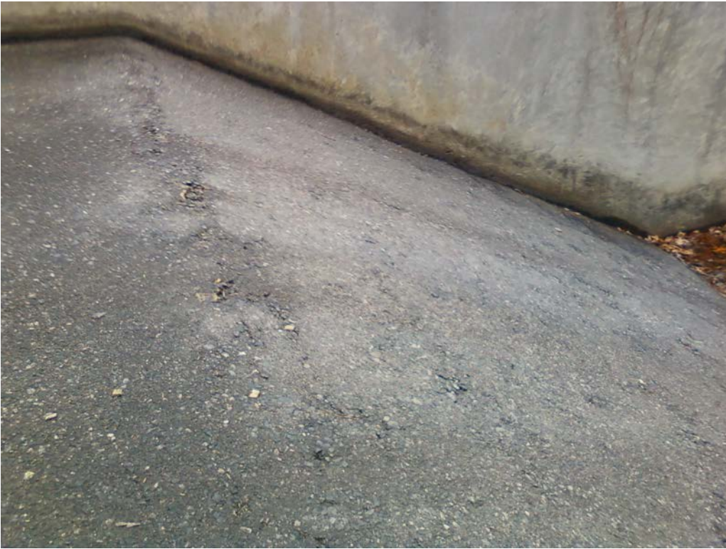
Photo 21c – The break in the spillway weir crest showing signs of mild weathering and surface erosion.
