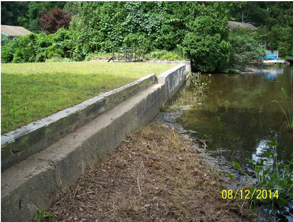
Photo 4 – A view of the upstream face from the left abutment. Note the spillway is in the upper center of the photo and that the right abutment is covered in trees and brush.
