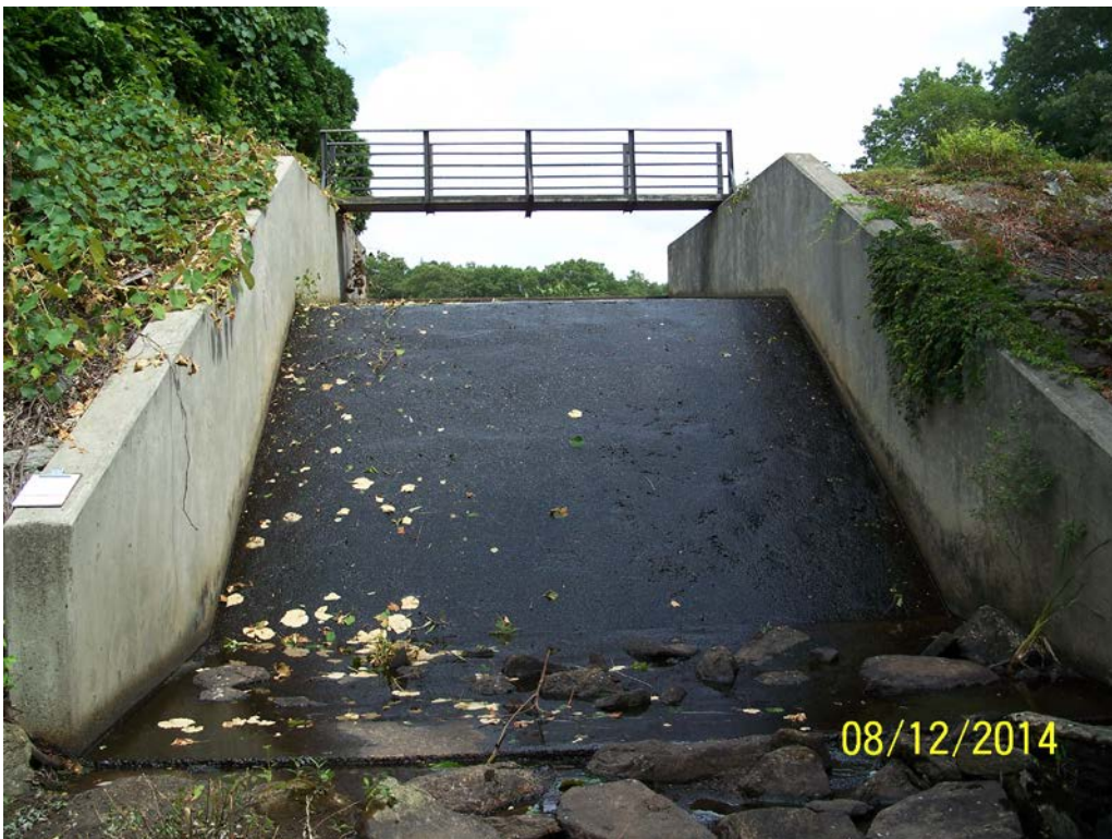
Photo 10b – Another view of the spillway from downstream with particular emphasis on the cover along the right spillway embankment slope area.
