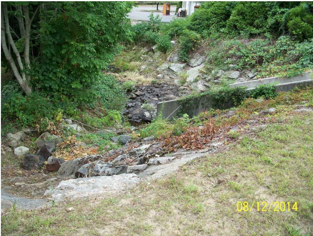
Photo 8a – The downstream face of the embankment to the left of the spillway as seen from the top of the dam, adjacent to the house (to the left of the photo – see Photo 8c). Note heavy vegetative growth along the toe and right embankment areas, as well as small brush growth within the downstream riprap slope.
