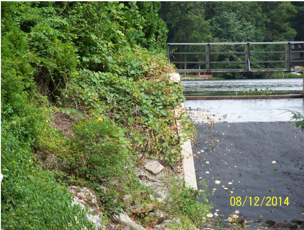
Photo 21g – The tree and brush cover along the right abutment embankment slope and dam crest.
