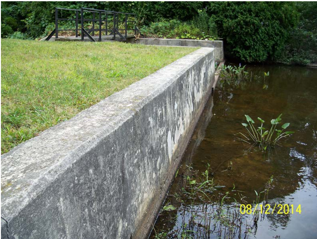
Photo 1a – An overview of the dam taken from the left (east) abutment. The spillway is at the upper center of the photo; the spillway bridge is visible at the top left center.
