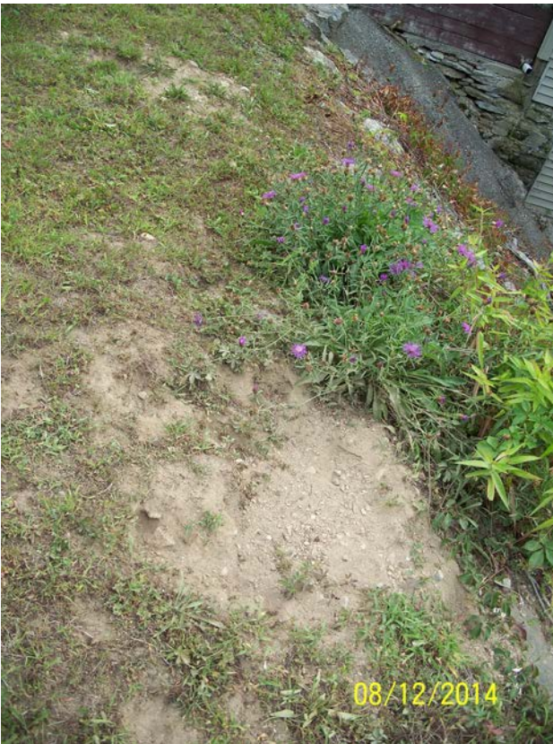
Photo 21d – Crest of the downstream embankment, left of the spillway and right of the house showing an area devoid of vegetation.
