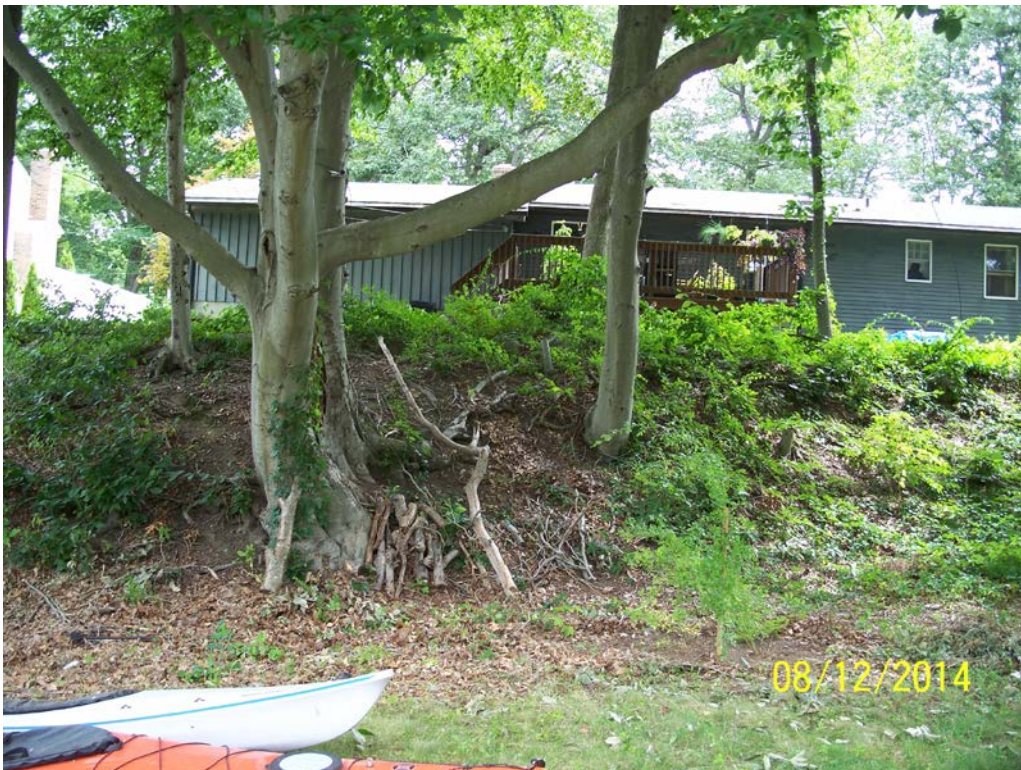
Photo 21j – Trees at the left abutment area within the 25-foot clearance zone.
