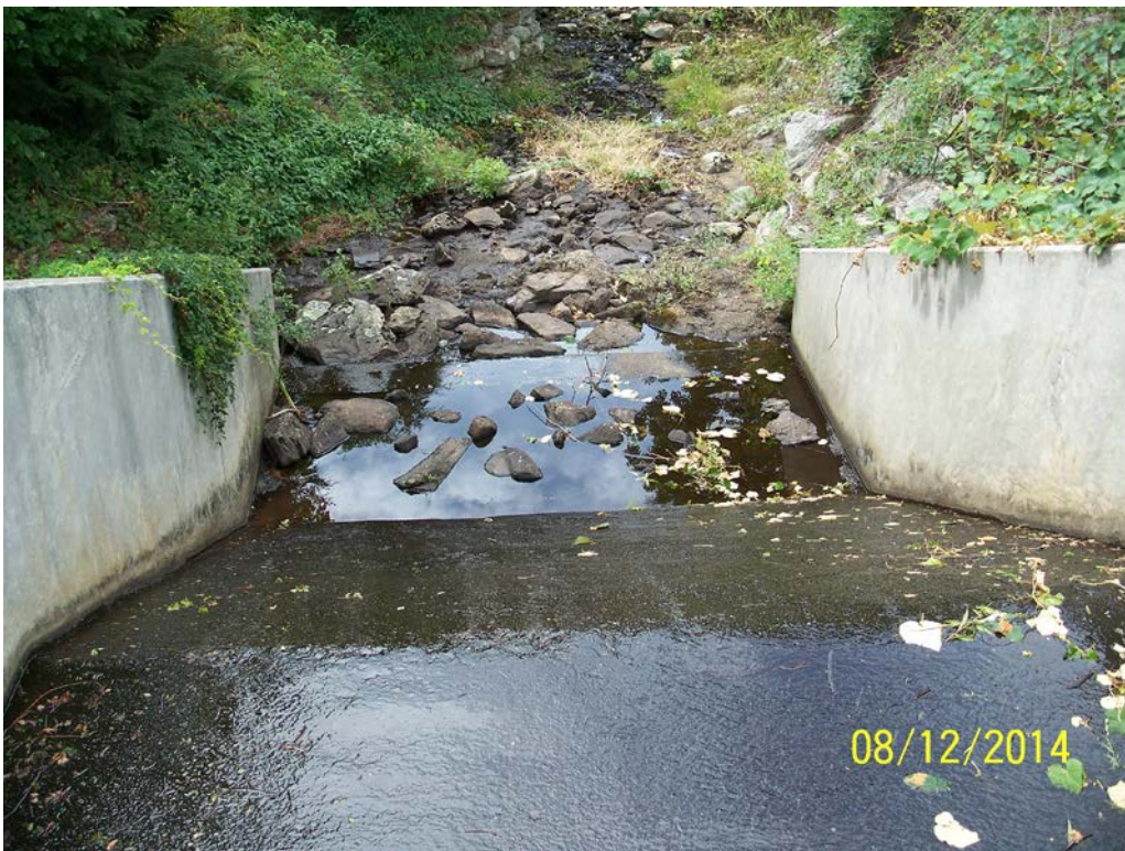
Photo 14 – The stilling basin at the lower end of the sloped spillway discharge channel. The riprap at the base was in stable condition.
