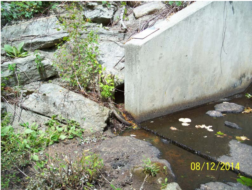
Photo 21i – The end of the right downstream spillway training wall, at the exit of the right toe and spillway underdrain discharge. Roots in this area need to be removed to allow free discharge of flow from the drains.
