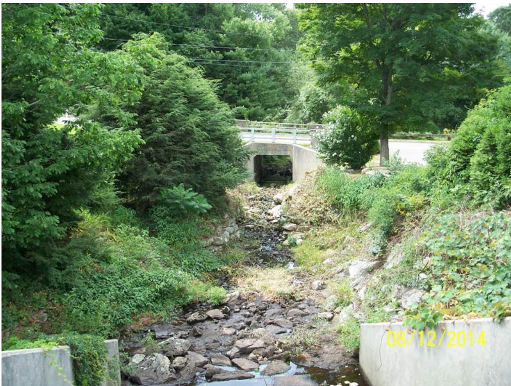
Photo 21h – The vegetative cover along the toe and downstream channel side slope areas.
