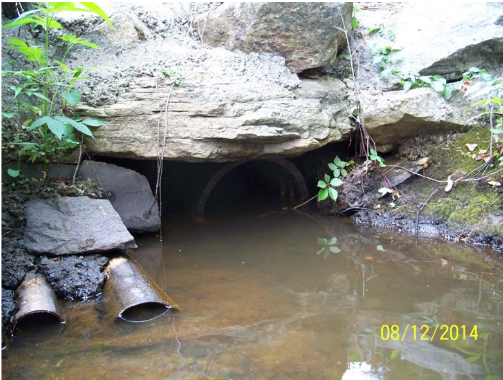
Photo 19 – The low level outlet area at the base of the left embankment adjacent to the spillway, showing the ductile iron outlet pipe and PVC discharge pipes for toe drain and spillway underdrain pipes. The intake area on the upstream side was submerged beneath pond level and could not be accessed at the time of inspection.
