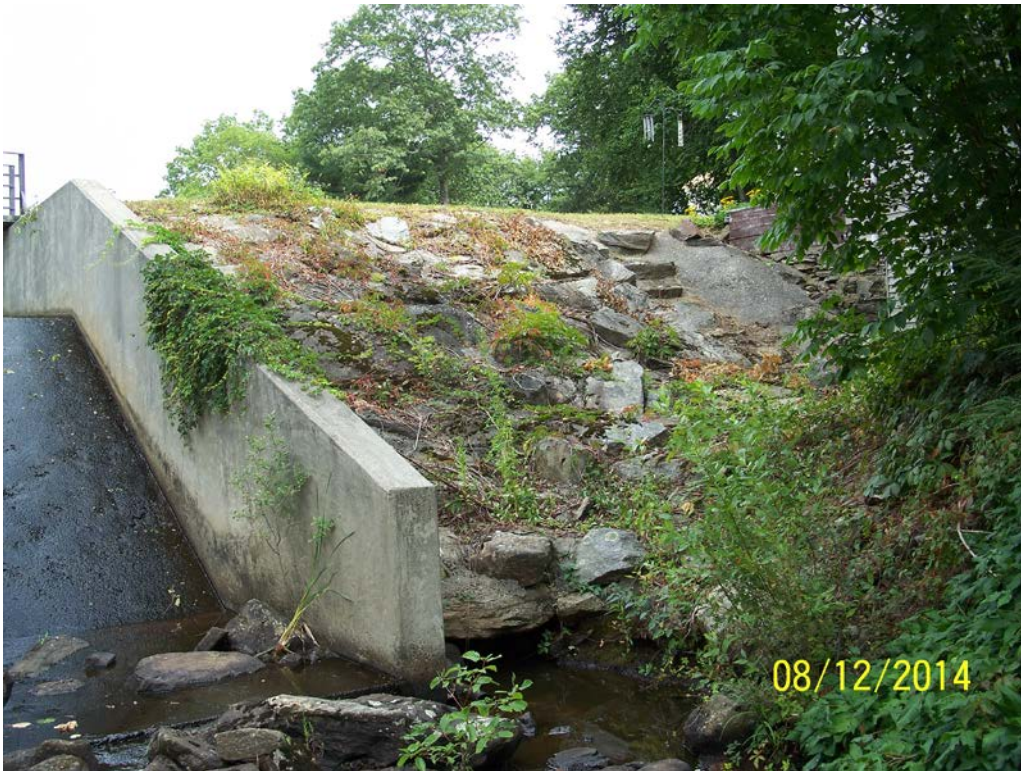
Photo 12b – Another view of the left spillway training wall from the center of the downstream channel. (See also Photo 5a for a view of the left training wall at the footbridge crossing).
