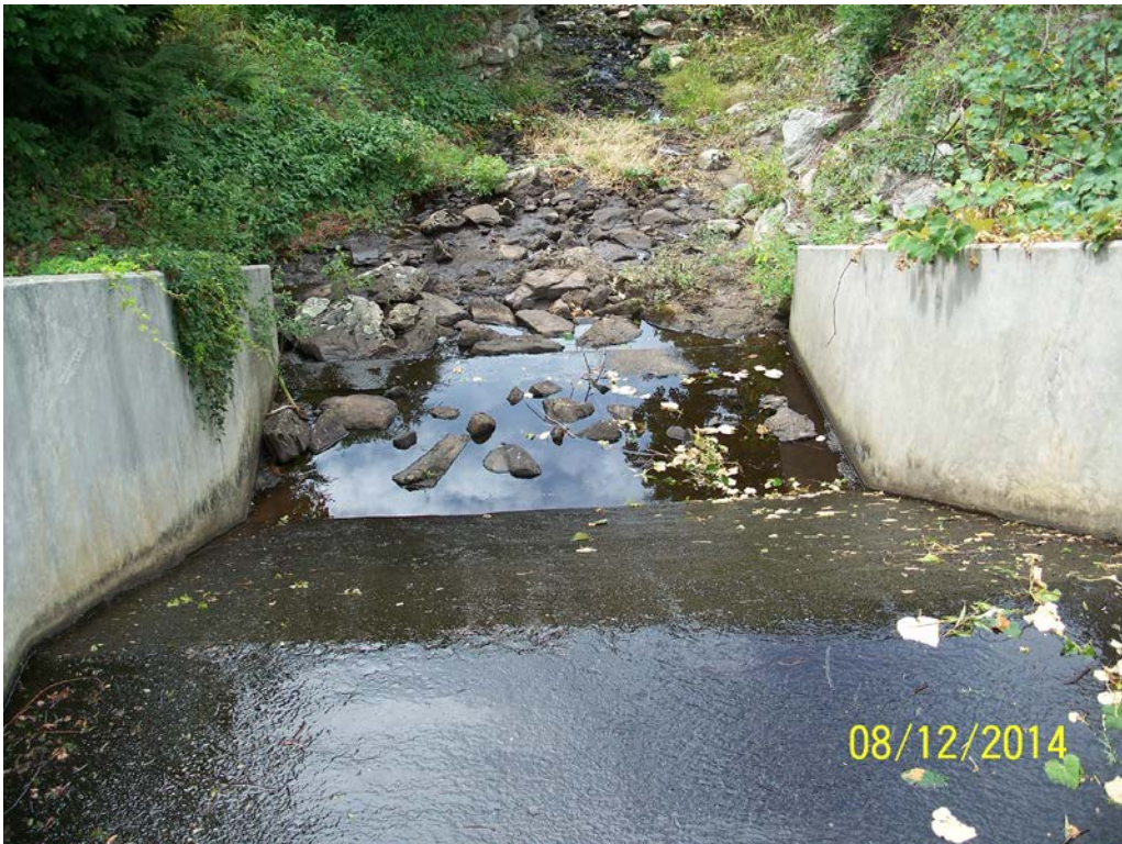
Photo 9 – The spillway looking in a downstream direction from atop the spillway footbridge on the upstream end.
