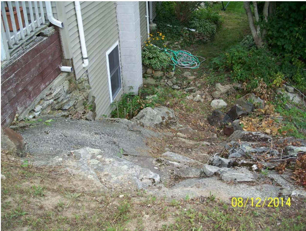
Photo 8c – Another view of the downstream slope to the left of the spillway, taken from atop the left embankment crest. (See also Photos 6 and 7b for views of the house situated on the left downstream embankment.)
