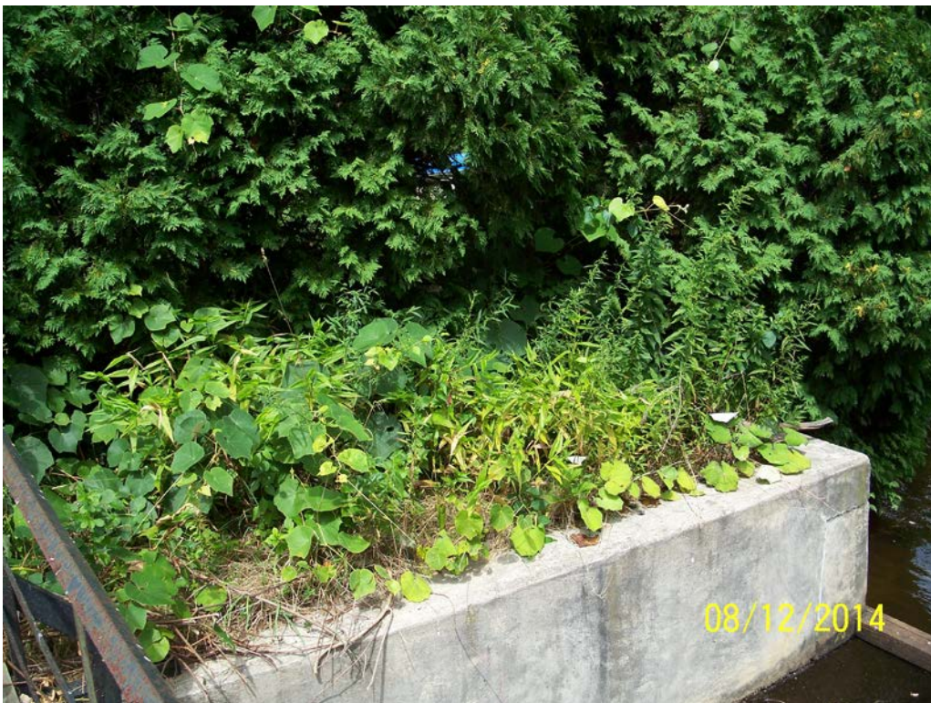
Photo 11b – A close-up of the upstream end of the right spillway training wall.
