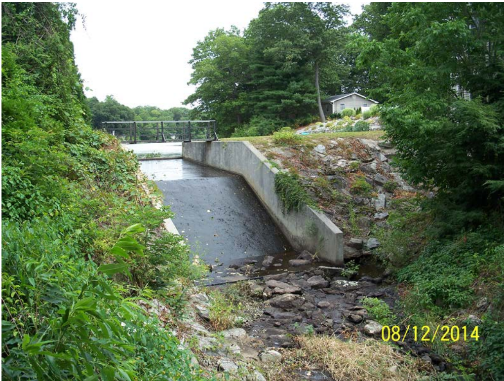
Photo 2 – Overview of the dam from the right downstream channel embankment looking toward the spillway and left embankment area. Because of the heavy vegetative cover, a more encompassing overview was impractical.
