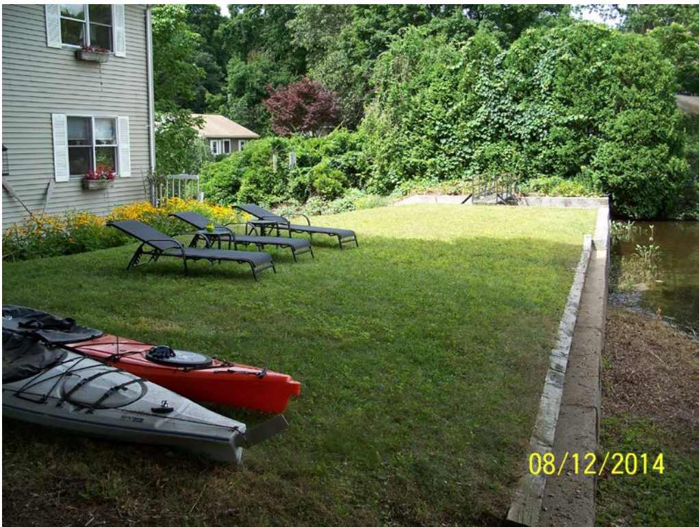
Photo 6 – An overview of the dam crest from the left abutment area. Again, note the house location with respect to the left embankment.
