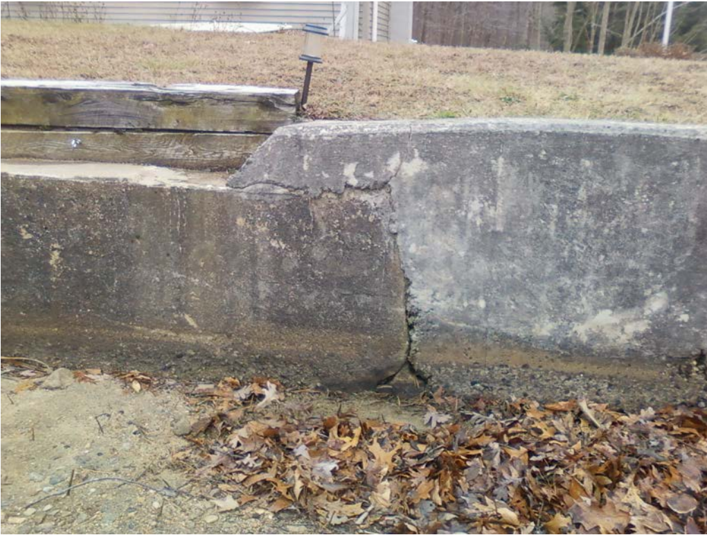
Photo 21a – The left upstream embankment wall showing minor crack and joint opening.
