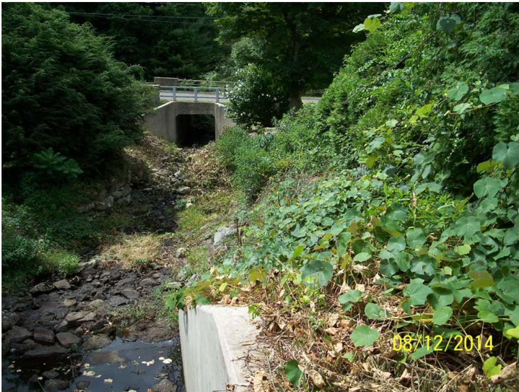
Photo 7a – The downstream face as seen from atop the right abutment area. The spillway is at the left bottom of the photo. Note the extensive vegetative growth along the right abutment and right downstream slope.
