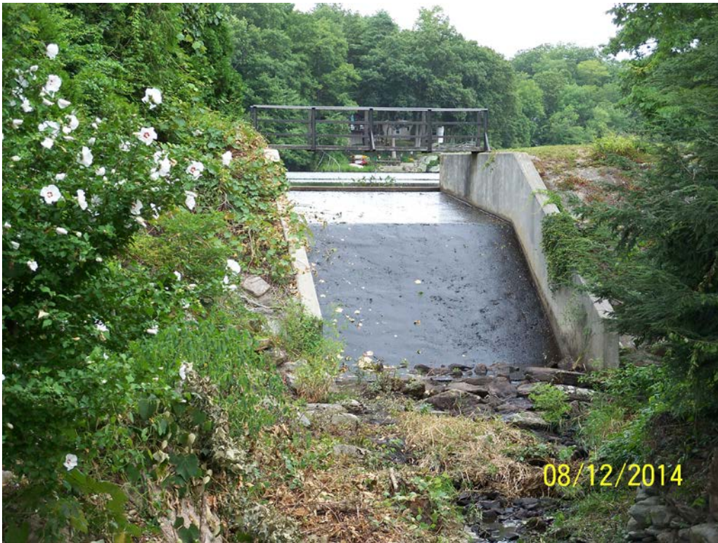
Photo 10a – The spillway as seen from the downstream channel. Note tree and brush cover along both sides.
