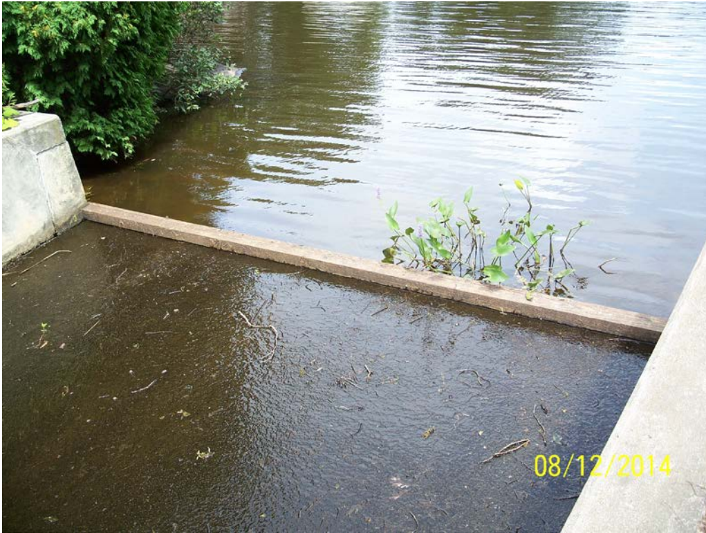
Photo 13 – An overview of the spillway weir, as seen from the left training wall looking upstream.
