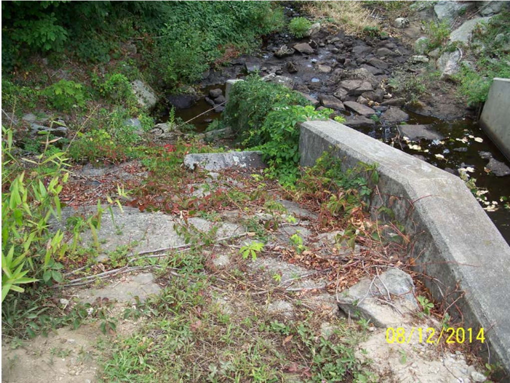
Photo 12a – An overview of the left spillway training wall; this wall is in generally good condition.
