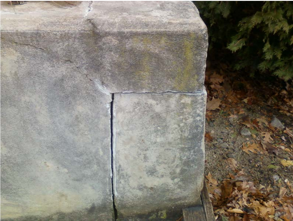
Photo 21b – Minor cracking and joint opening at the right upstream corner of the right spillway training wall. These should be cleaned and filled with appropriate repair materials.
