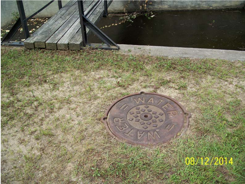
Photo 16 – The exterior of the valve chamber for the low level outlet pipe.
